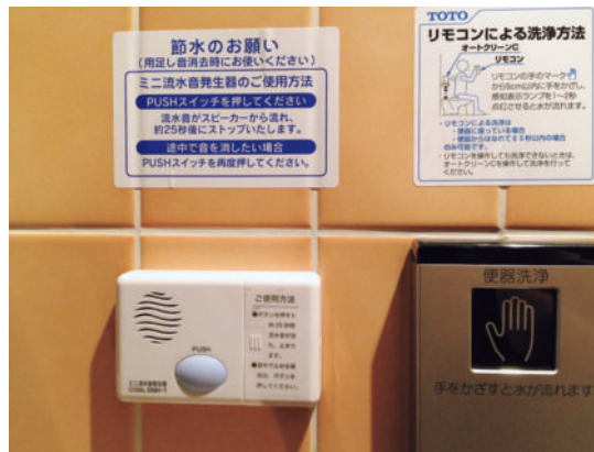
Figure 4 An example of the device on the wall of a hotel toilet. Above the device a notice has been placed which asks women to cooperate with water conservation and use the device if they want to drown out the sound when they use the toilet.
